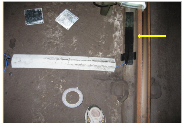
FBG Strain Sensor installed on track
